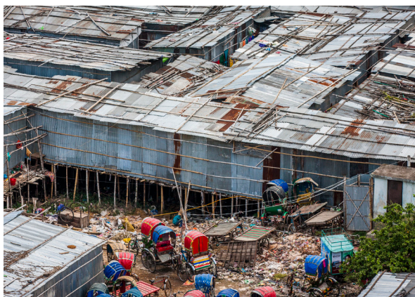
Dire living conditions in slums: Slum residents face higher rent costs than decent housing. 13 Their access to public service such as water and electricity is even more limited and costly, with a majority controlled by slumlords. 14
