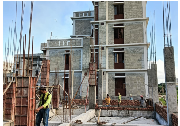
Multi-story building under construction in Chandpur District, as part of UNDP's NUPRP affordable housing.
