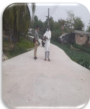
Image 3.20 Road constructed under the project (Length: 302 m. and Width: 3.5 m.), Chhotobaira, Shamshanghat, Khulna City Corporation
