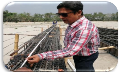
Image 3.4 Observation of Casting of Service Piles for Low Cost Housing in Gopalganj City (Building 3 and 4)
